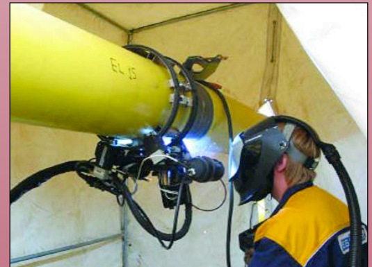
27cm (10") Gas Pipeline – Estonia
