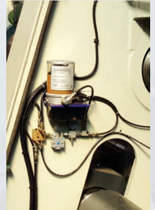
Automatic centralised lubrication.
